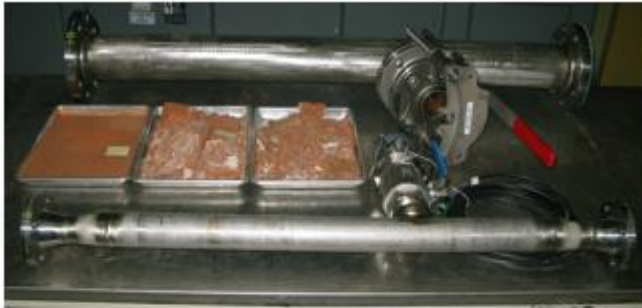
Unexpected "sludge" accumulation discovered
